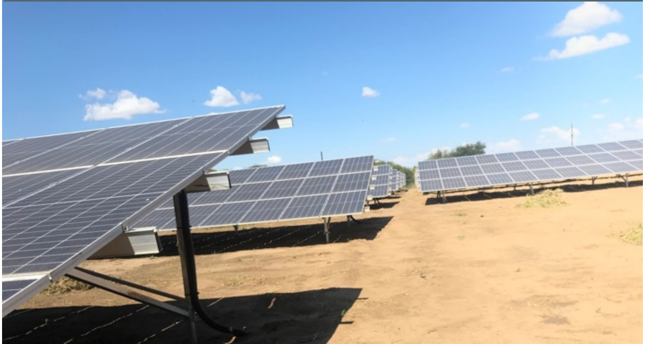
Solar panels installed at a plant in Beitbridge
