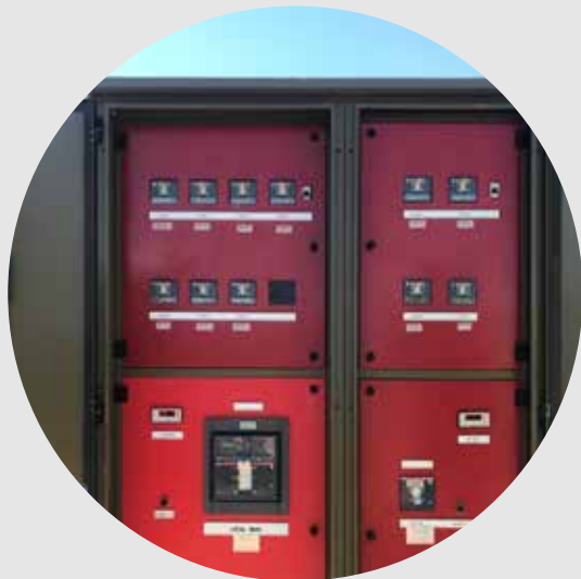
The inverters which convert and regulate power generated by the solar panels
