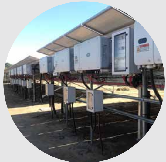
The regulator which regulates the power from the inverters and transfers it to the production plant
